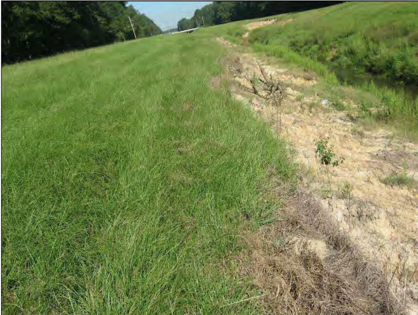
Inspect ID: EJFC_2016_a_0003 Title: USACE_CEMVK_EJFC_2016_a_0003_1.jpg Rated Item: 6. Erosion/ Bank Caving Caption: Rating: Acceptable; Remarks: RS Erosion 20' from the toe. The Levee Board is working on the solution for the problem.; Station_1: 30
