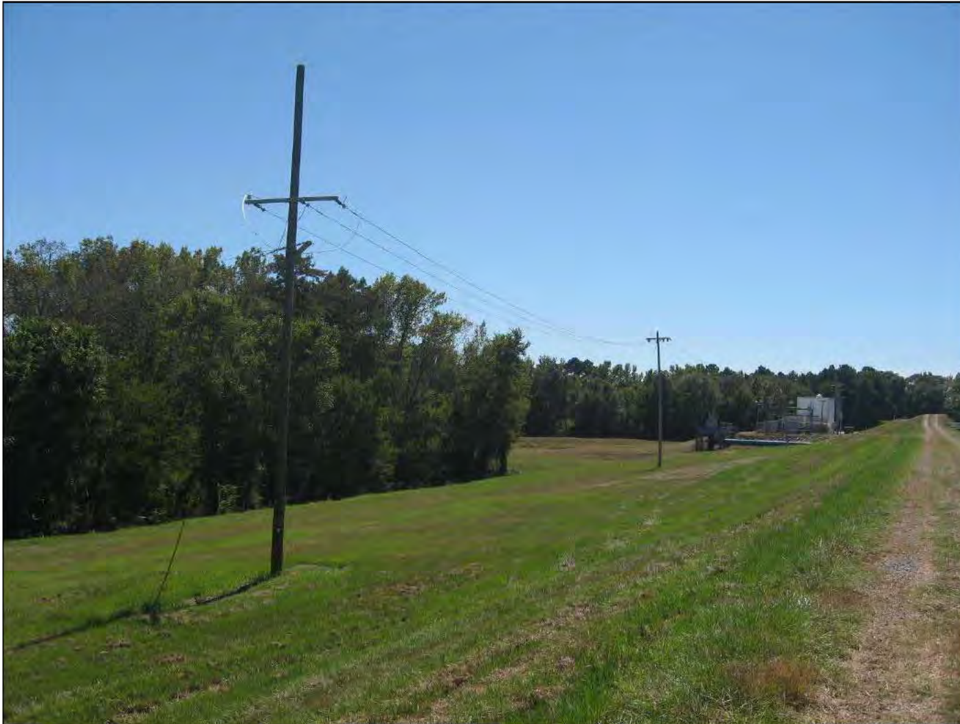
Inspect ID: EJFC_2016_a_0014 Title: USACE_CEMVK_EJFC_2016_a_0014_1.jpg Rated Item: 3. Encroachments Caption: Rating: Minimally Acceptable; Remarks: STA 408 Utility poles LS and RS within 40' of toe.; Station_1: 408
