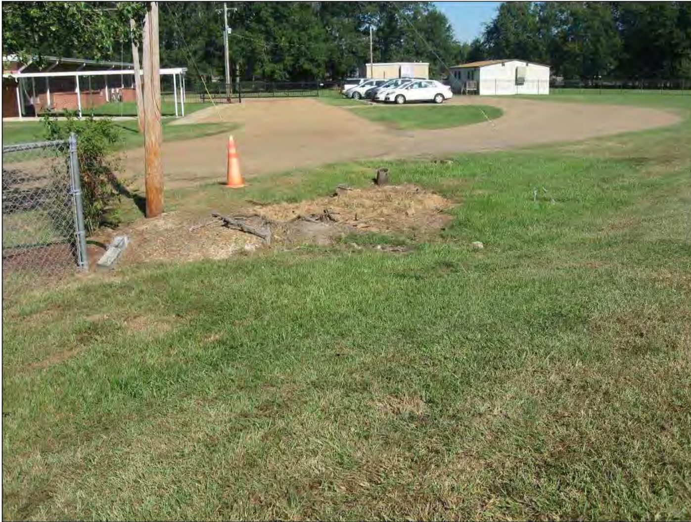
Inspect ID: EJFC_2016_a_0001 Title: USACE_CEMVK_EJFC_2016_a_0001_1.jpg Rated Item: 1. Unwanted Vegetation Growth Caption: Rating: Acceptable; Remarks: STA 0+00 Previously noted tree has been removed.; Station_1: 0+00
