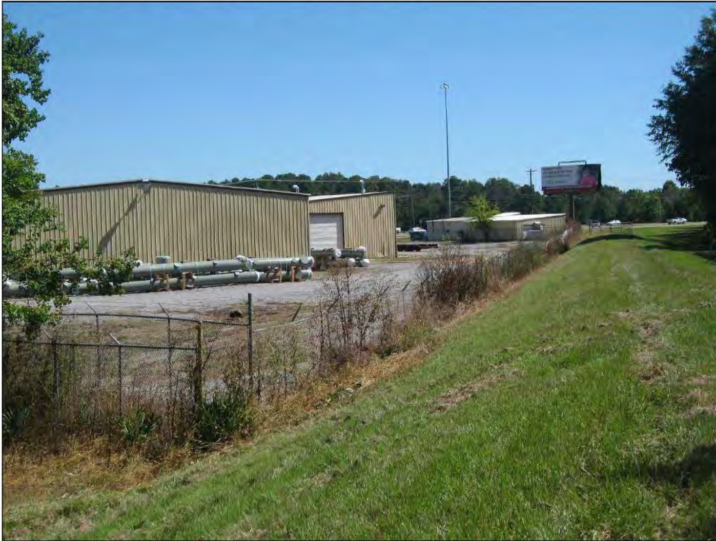
Inspect ID: EJFC_2016_a_0018 Title: USACE_CEMVK_EJFC_2016_a_0018_1.jpg Rated Item: 3. Encroachments Caption: Rating: Minimally Acceptable; Remarks: STA 515 LS Fence parallel along toe of levee in federal government/military compound.; Station_1: 515
