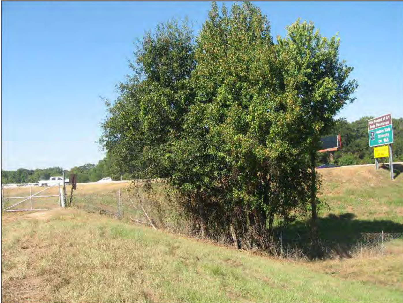
Inspect ID: EJFC_2016_a_0011 Title: USACE_CEMVK_EJFC_2016_a_0011_1.jpg Rated Item: 1. Unwanted Vegetation Growth Caption: Rating: Minimally Acceptable; Remarks: STA 320 vegetation in levee slope at intersection of I55 needs to be removed or will be rated U next year; Station_1: 320
