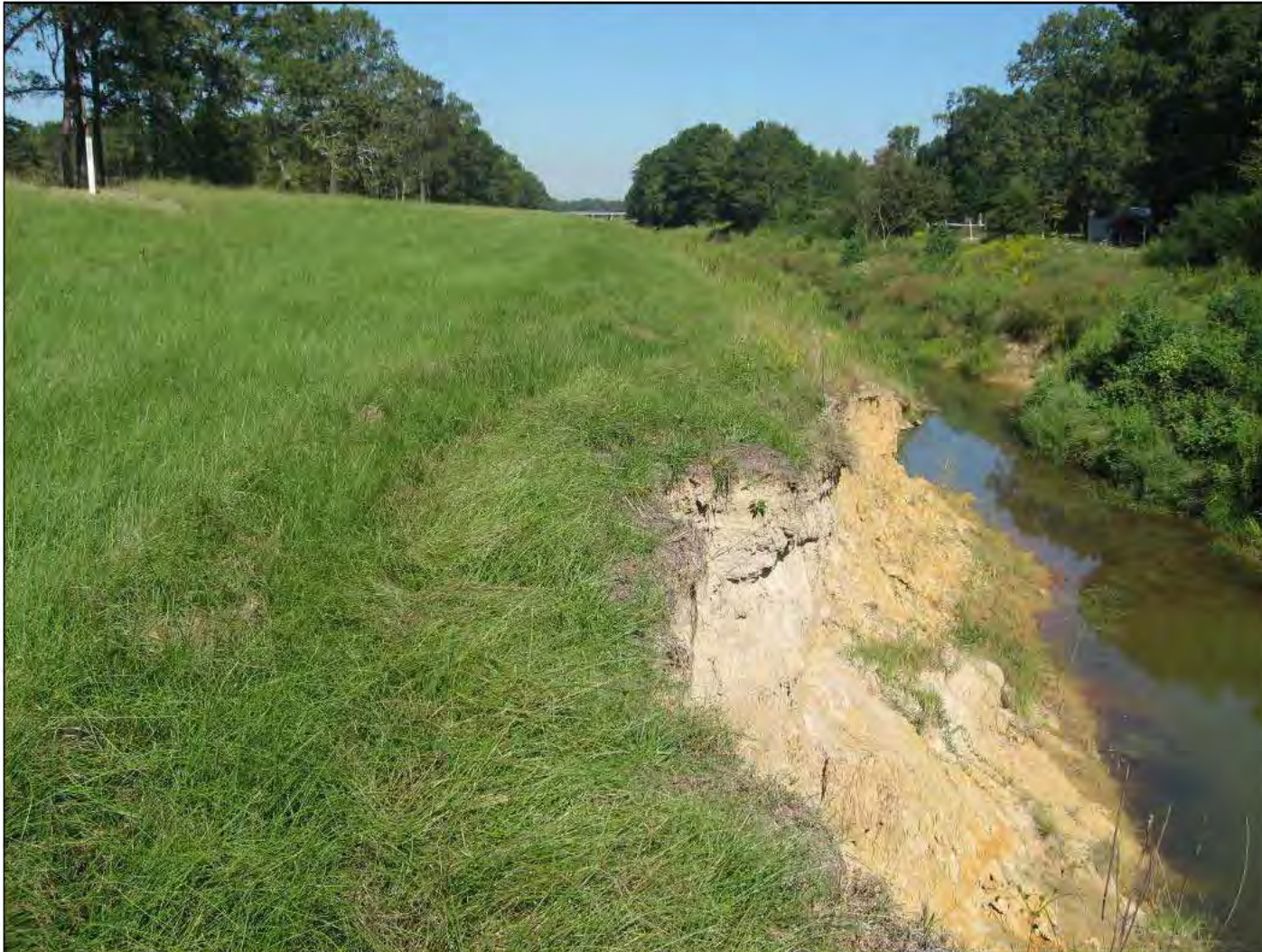
Inspect ID: EJFC_2016_a_0007 Title: USACE_CEMVK_EJFC_2016_a_0007_1.jpg Rated Item: 6. Erosion/ Bank Caving Caption: Rating: Acceptable; Remarks: RS Erosion about 30' from the toe.; Station_1: 47
