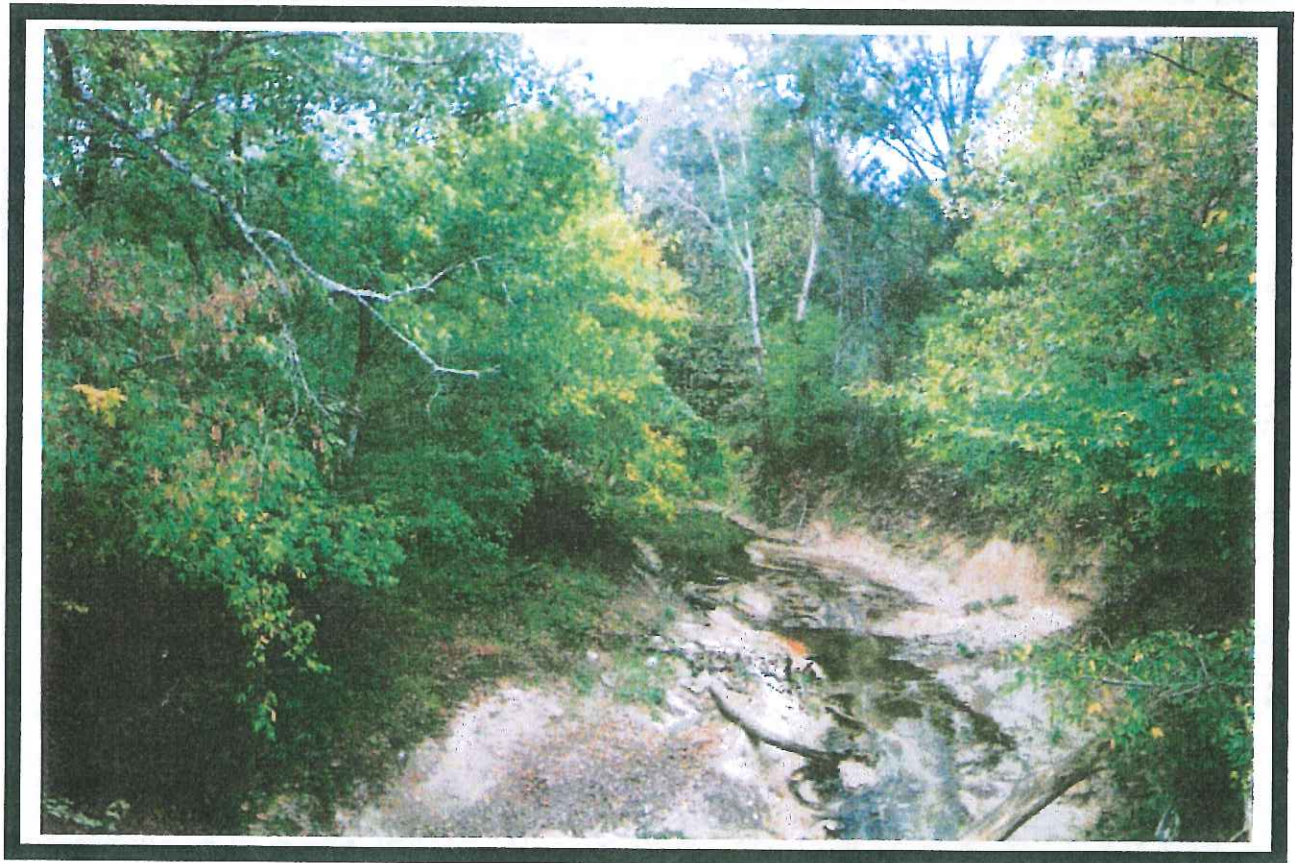
Figure 8. Caney Creek below Savannah Street sewage lagoons a. abandoned railroad trestle, b. steep and eroding bank line.
