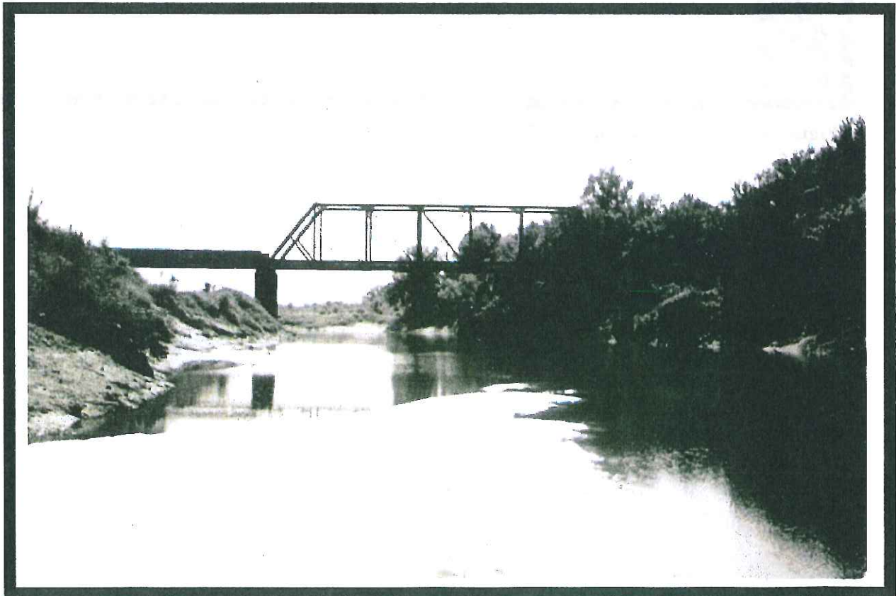
Figure 185. Illinois Central railroad at Hinds/Rankin Landing/Ferry (22-Ra-671); a. railroad bridge view east; b. view south.
