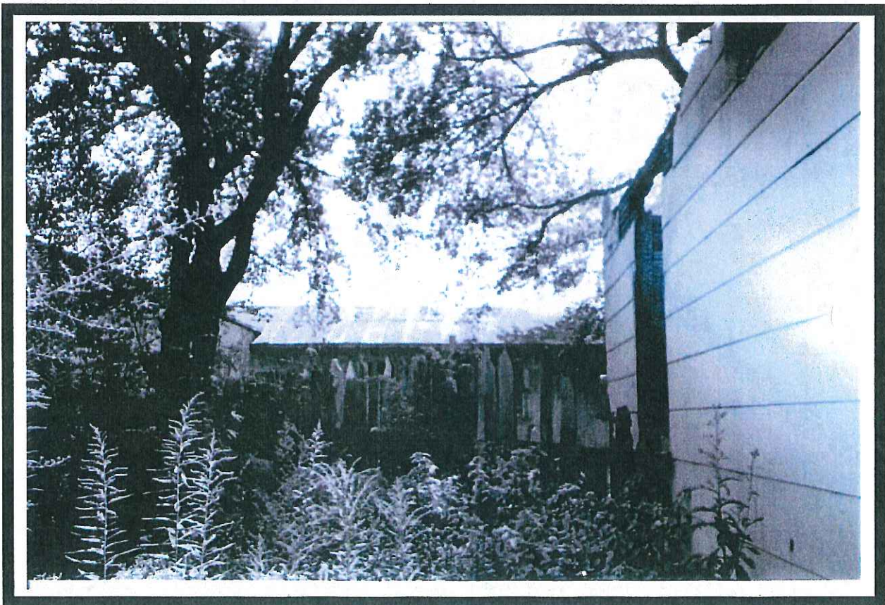
Figure 295. Farrish Street burned shotgun house; a. piers and door; b. picket fence.
