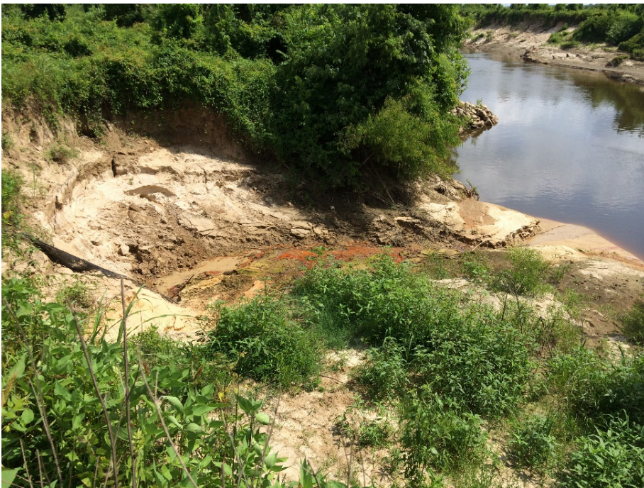
Picture 14 – Erosion and Seepage Area along Pearl River
